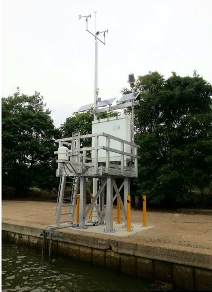
Elevated Water Level Station
